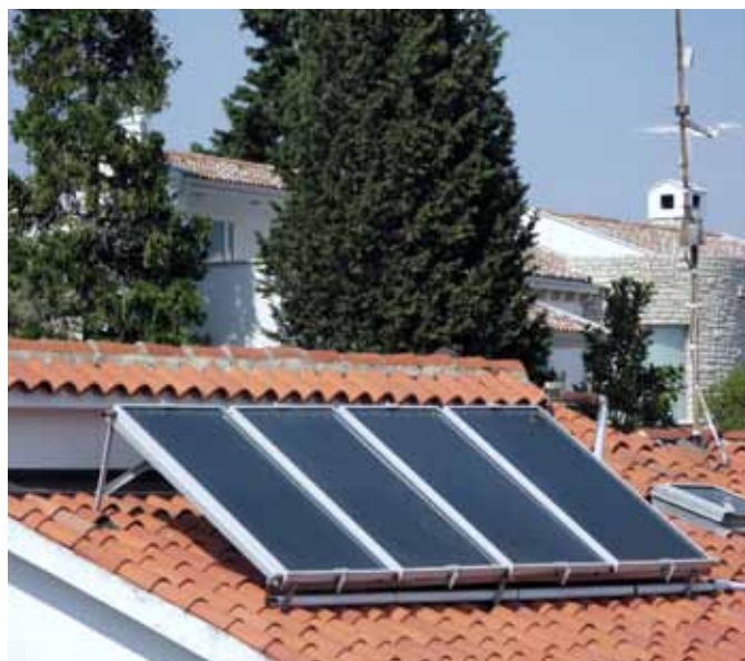
Illustration 4. Solar water heaters on a roof
